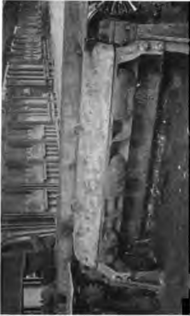
Fig. 2. Trial Installation of Cast-Iron Gear Shield for Roller Train. (National Tube Company.)*
